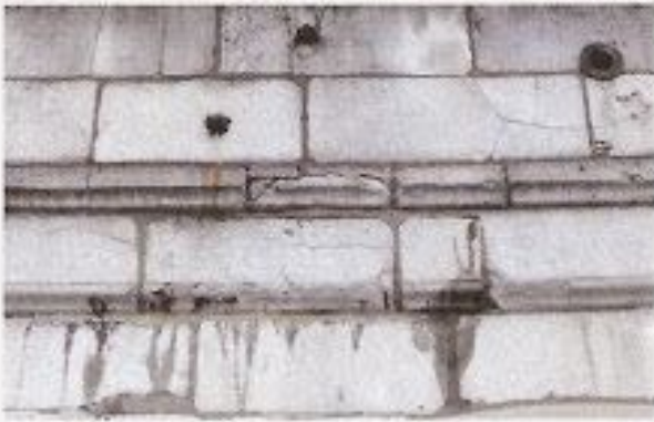
Staining and parapet cracks
