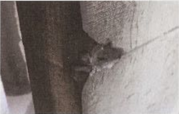
Damage by rusting cramp
