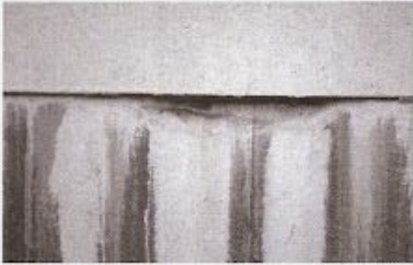
Rusting cramps damaging ashlar face
