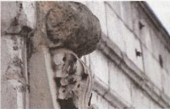
Parapet cracks; sculpture erosion; inappropriate pointing
