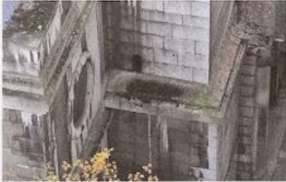
Heavy staining and bird pollution
