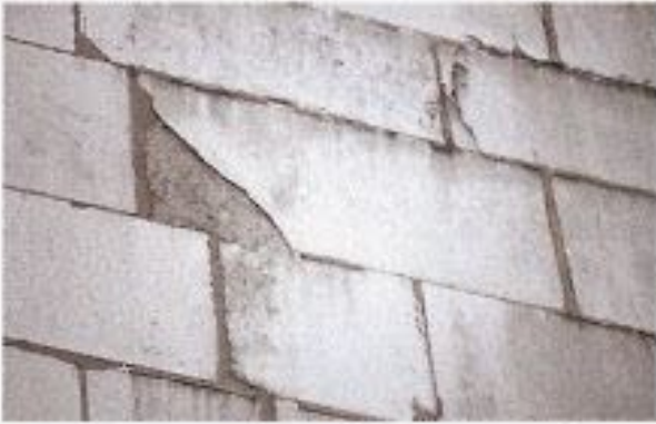
Rusting cramps damaging ashlar face
