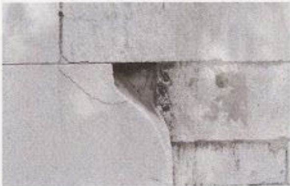
Ferrous cramp damage
