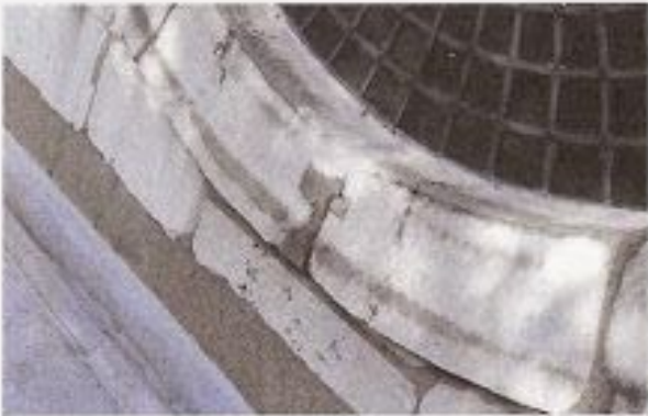
Cement mortar fillet; ferrous cramp damage
